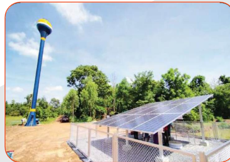
Solar Pumping System >1,000 Sites
