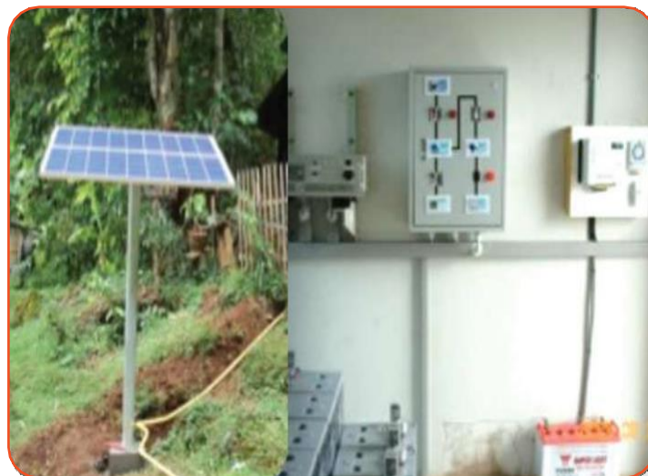
Solar Off-grid System 55 MW
